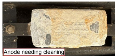
Anode needing cleaning
