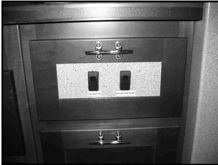
Pressure pump switch
