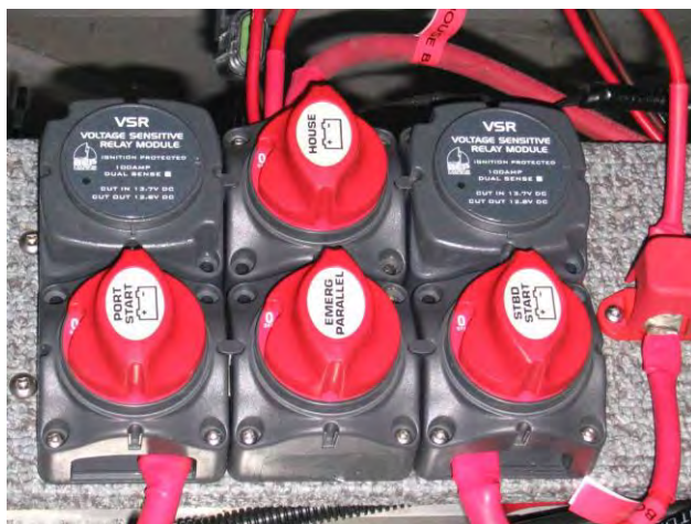
Three bank battery system switches
